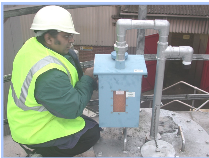
615 Tank Vent Dryer installed with over pressure relief valve protection
